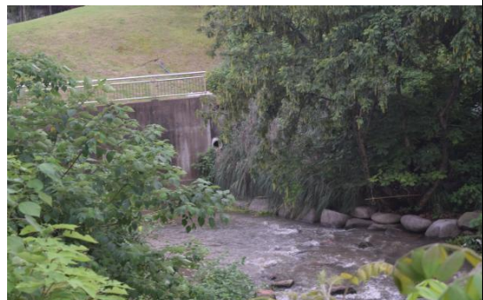
防洪排涝区防护
